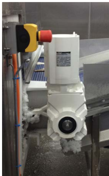
The Bauer gear motors work well at minus 43^{\circ}\text{C} .
